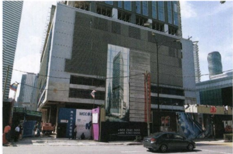
Being main contractors, the Chinese companies still need to farm out jobs to local subcontractors as it is very unlikely that they could do everything on their own
