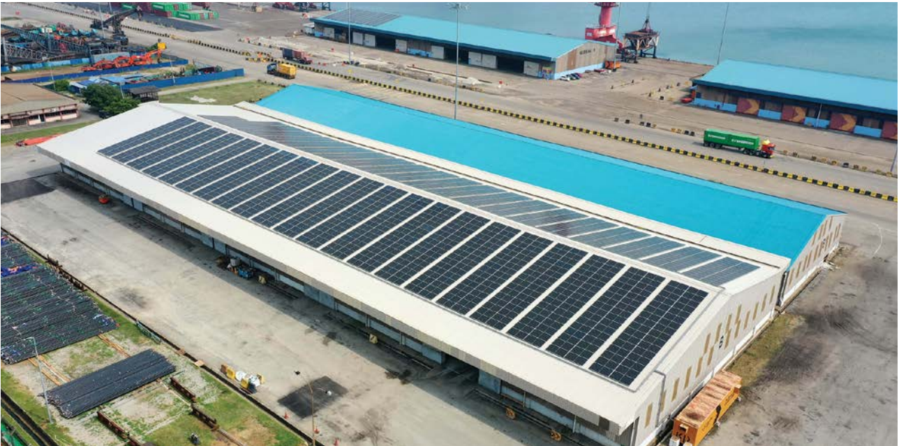
Solar PV panels installed at Kuantan Port
