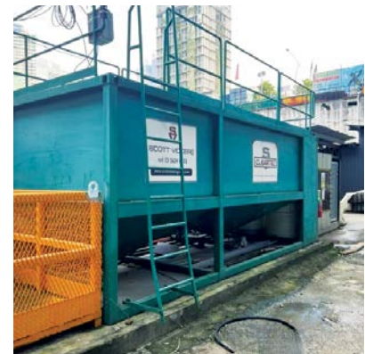
Water treatment system at TRX Residences site in Kuala Lumpur
