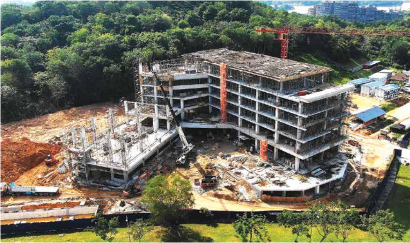
SMART IBS solution employed at a data centre project, Cyberjaya
