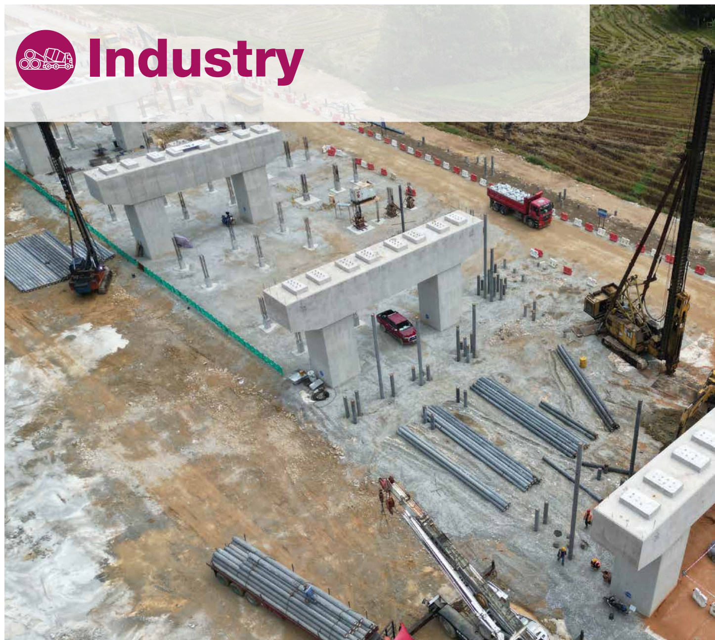
ICP piles used in the East Coast Rail Link project, Kota Bharu
