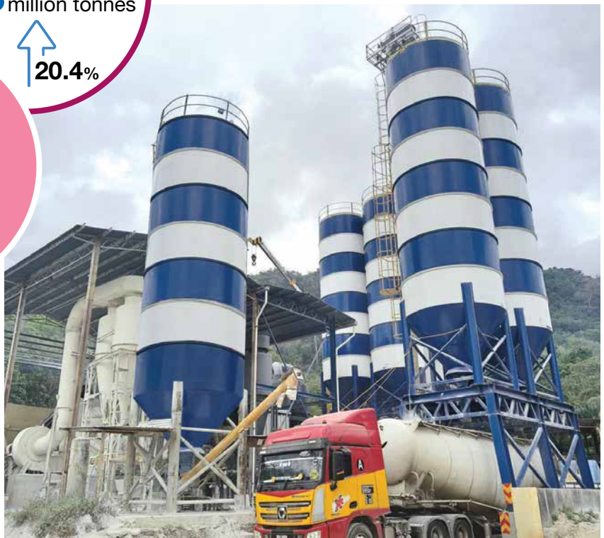
Grinding mill at Raub, Pahang
